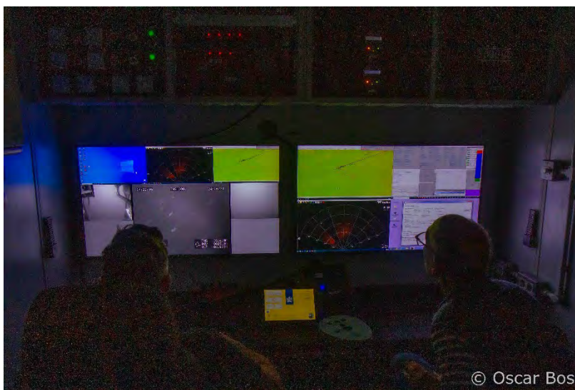
Figure 10. ROV control room.
