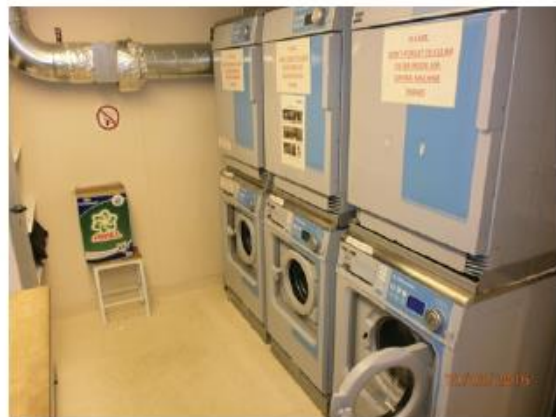
A laundry with three industrial washing machines and dryers.
